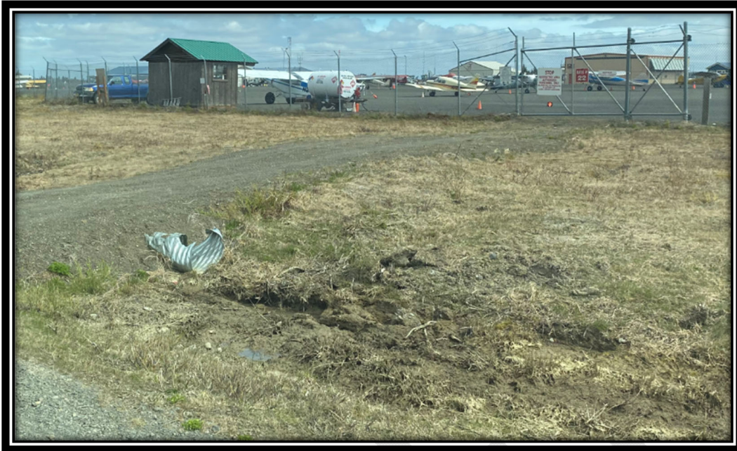
Figure 8: Damaged Culvert under GA Apron Access Driveway
