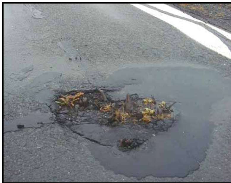
Figure 4: Pothole in Runway 15-33
