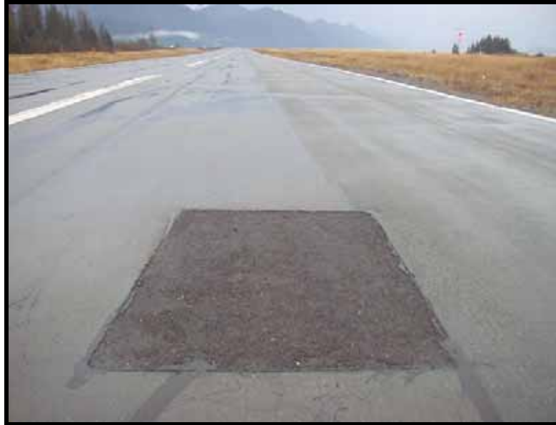
Figure 3: A Recent Patch on Runway 12-30
