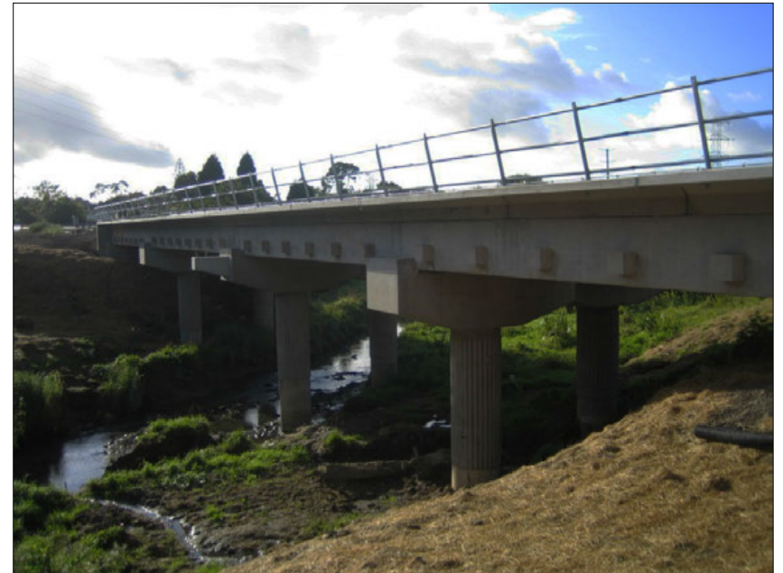
Figure ALT17. Example of similar bridge (KiwiRail Whau Creek Bridge, Auckland, New Zealand) under construction (photograph courtesy of HEB Construction Limited).
