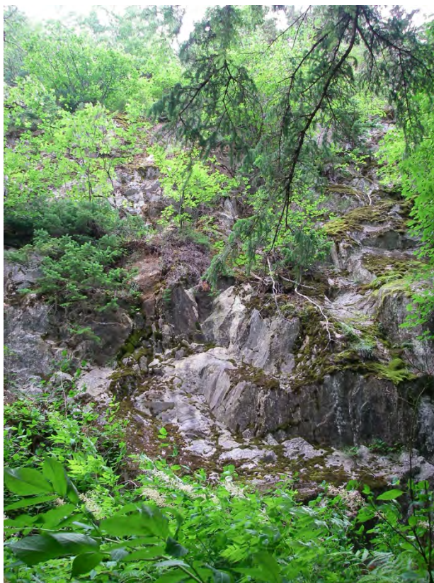
RF42. View east/upslope at rockfall hazard.
