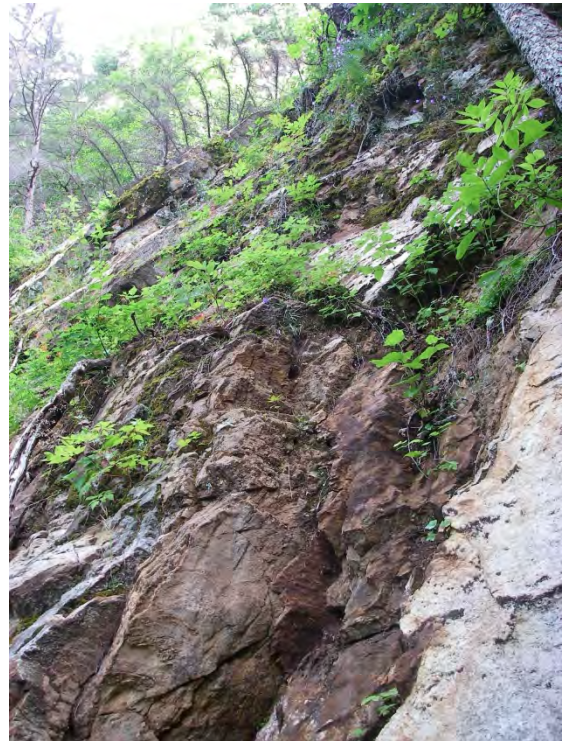
RF49. View north/up alignment across rockfall hazard.
