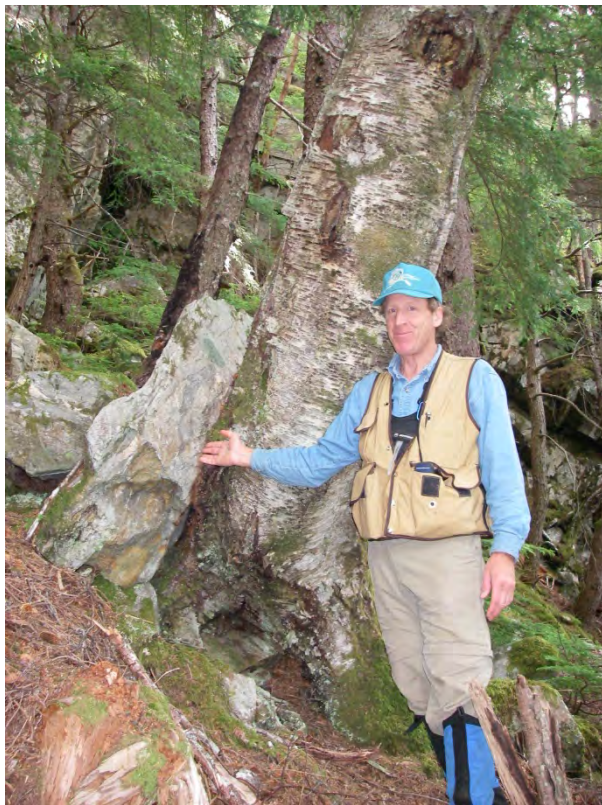
RF43. View south/down alignment at rockfall hazard, recently deposited boulder embedded into 2 ft diameter birch tree.
