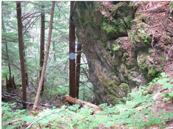
RF46. View northwest (up alignment and downslope) at rockfall hazard area.
