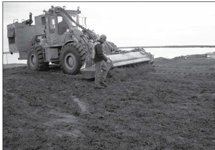
Supervised soil and fiber blending process. The blending time was approximately three hours.
