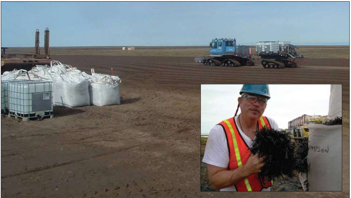
The 275 gallon plastic totes of synthetic binder and bags of geo fiber.
