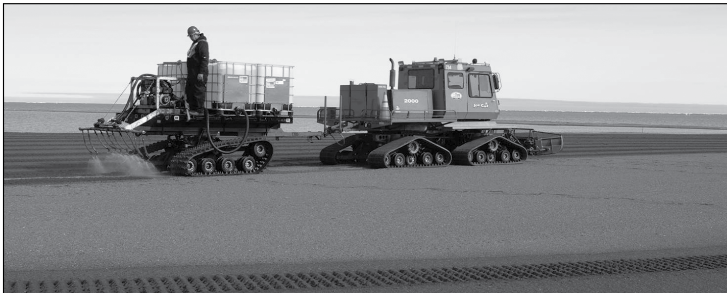
First synthetic fluid application. Tracked equipment was used for the application due to lack of surface bearing for conventional wheeled vehicles.
