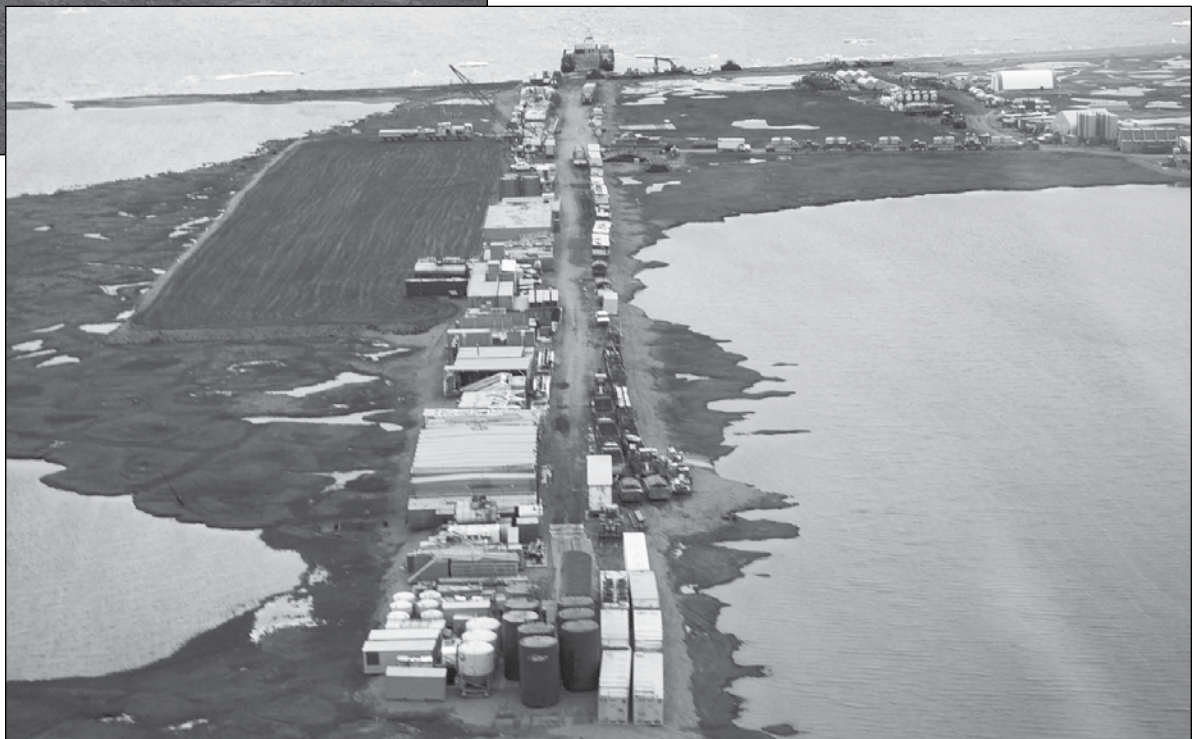
Leaving the pad ready for work. Synthetic fluid and geo fiber application took three days with a base crew of five people. Stabilization cost approximately $1.95 per square foot.
